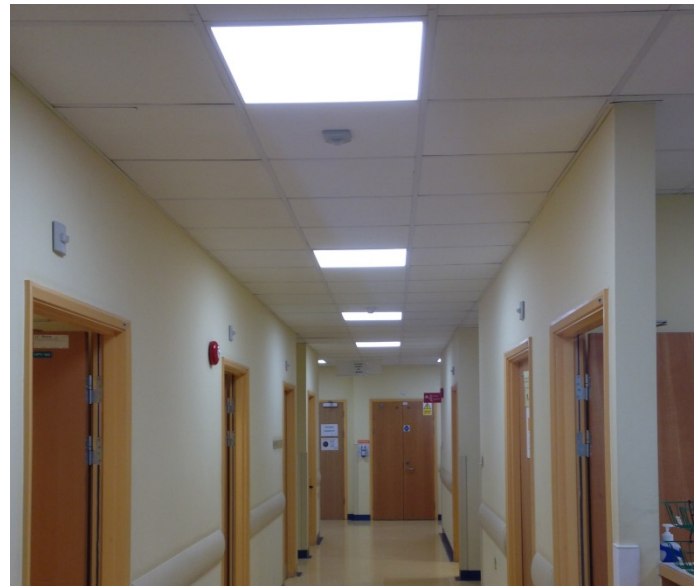
New lighting in wards at Maidstone hospital
